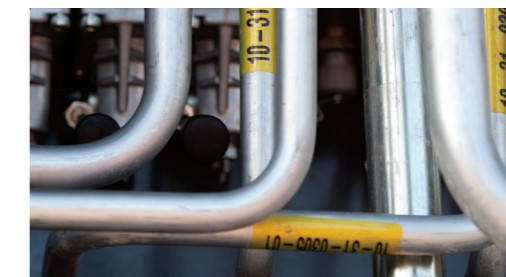
Steel pipework for better heat dissipation
